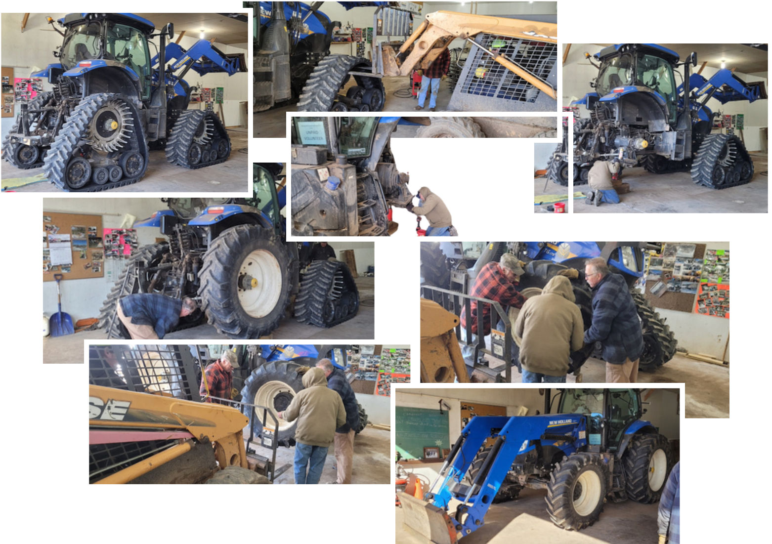
With the change of seasons it becomes necessary to either install or remove the Soucy Tracks on our tractor. Here are Doug Bruner, Jim Becker, Jim McDowall and Brent Ringlein putting the tires back on the New Holland getting it ready for summer grading. Trevor Thompson is operating the skid steer.
